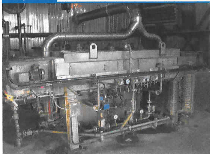
Filter press complete with vapor collection system.
